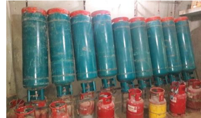
Cylinders being illegally filled
